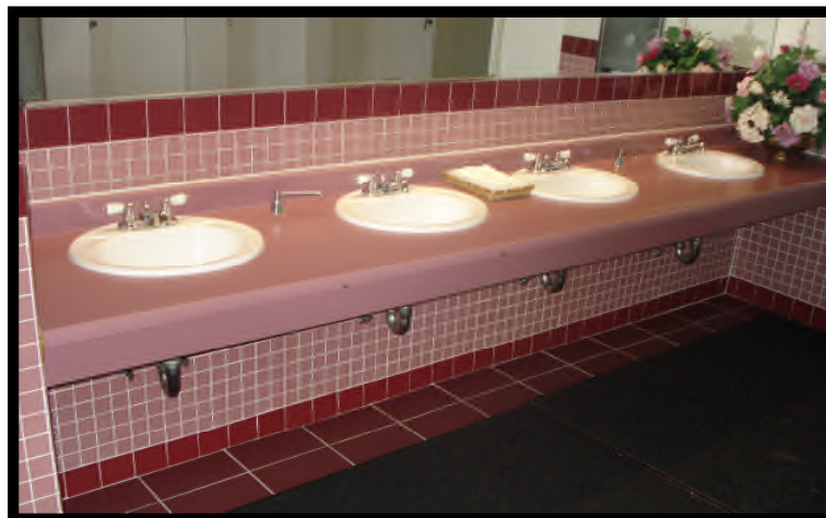
Fort MacArthur, Pacific Crest & Pacific Heights, San Pedro, CA Bldg. 403: Replaced Tile and Subfloor in Men's Restroom Call Henry, Inc. - Jose Perez (310) 597-3323
