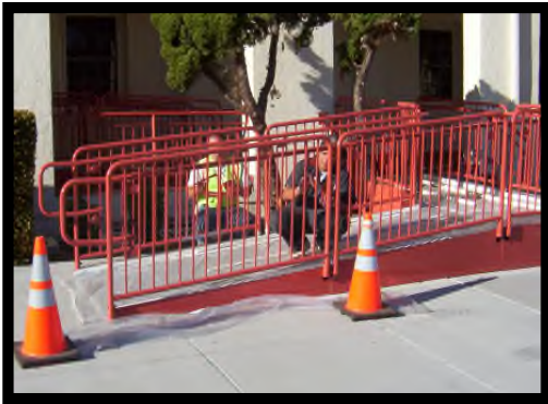
Fort MacArthur, San Pedro, CA Installed Handicap Ramps & Handrails; Converted Manual Doors to Automatic Call Henry, Inc. - Jose Perez (310) 597-3323
