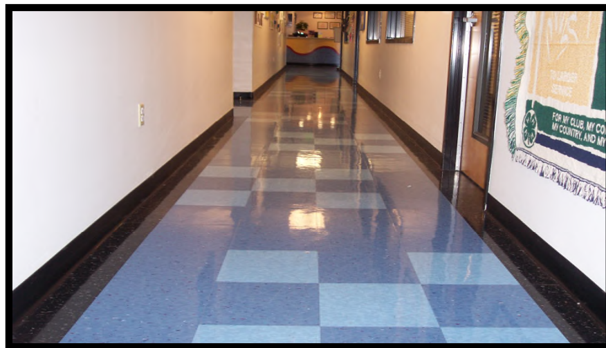
Fort MacArthur, San Pedro, CA Youth Center: Replaced VCT Tile Floor and Cove Base; Repaired/Replaced Subfloor; Painted Interior Walls Call Henry, Inc. - Jose Perez (310) 597-3323
